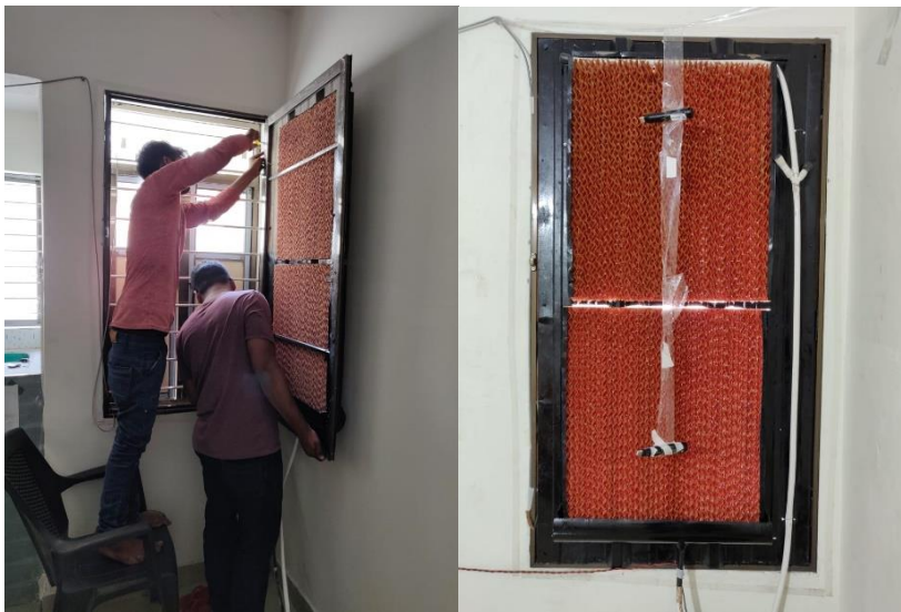
Figure 9: Centrally assisted night ventilative cooling with entering through windows: test of direct evaporative cooling of a window covered with a low-pressure loss wet pad.
